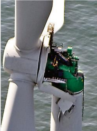
Damaged nacelle „alpha ventus“ in april 2018
